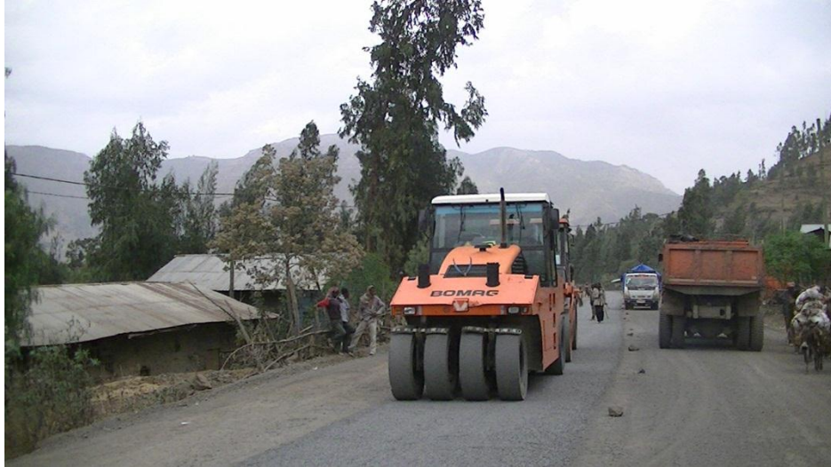
Figure 4-4 Rolling in progress by the use of both a pneumatic roller and the loaded tipper truck
