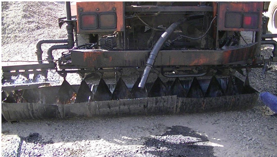
Figure 4-1 Checking of the nozzles prior to sealing operations and spraying of binder
