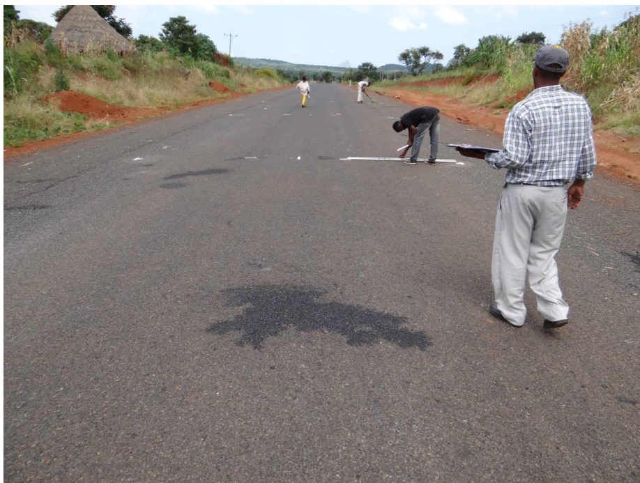
Figure 2-12 Spillage of petroleum products on the surfacing
