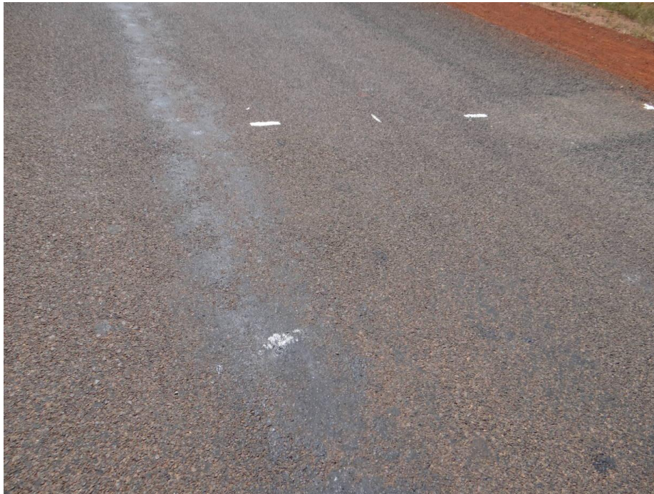
Figure 2-11 Short length of bleeding on the inner lane of a curve
