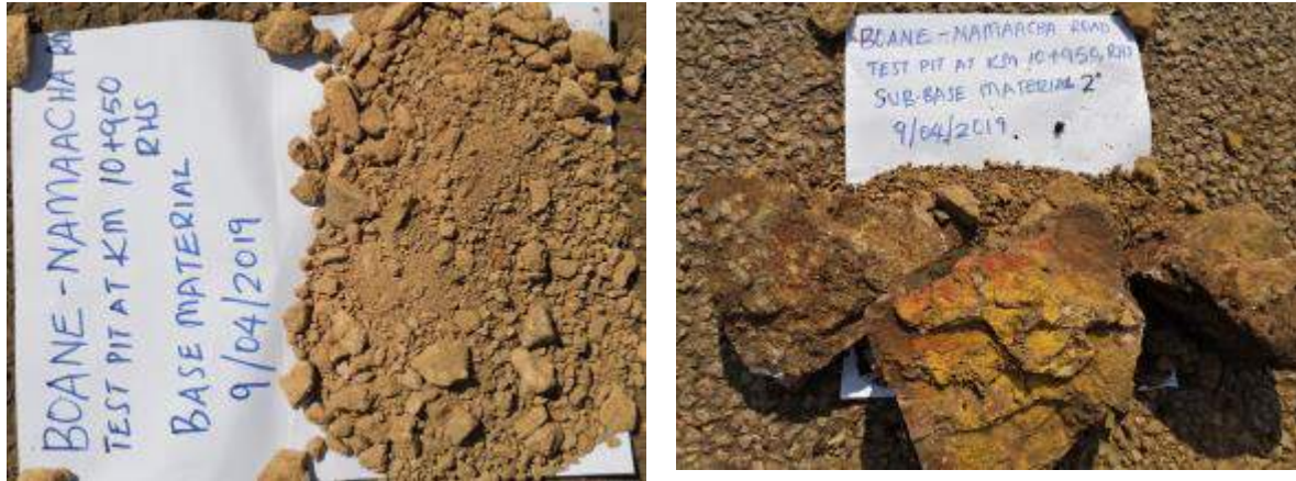
Figure 9 Base course material and cobbles for sub-base observed on Section 3 of Boane – Namaacha road
