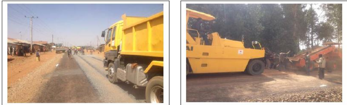
Figure 12 Rolling in progress by the use of both a pneumatic roller and the loaded tipper truck.
