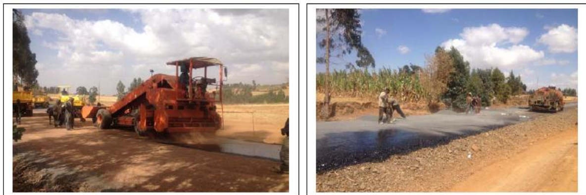
Figure 11 Self-propelled chipspreader in operation and the sprading of aggregate by the use of labour.
