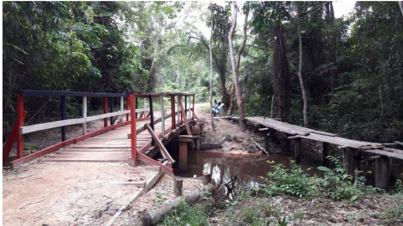
Picture 2 - Newly constructed track bridge next to the old footbridge near Gogein, Nimba County, Liberia
