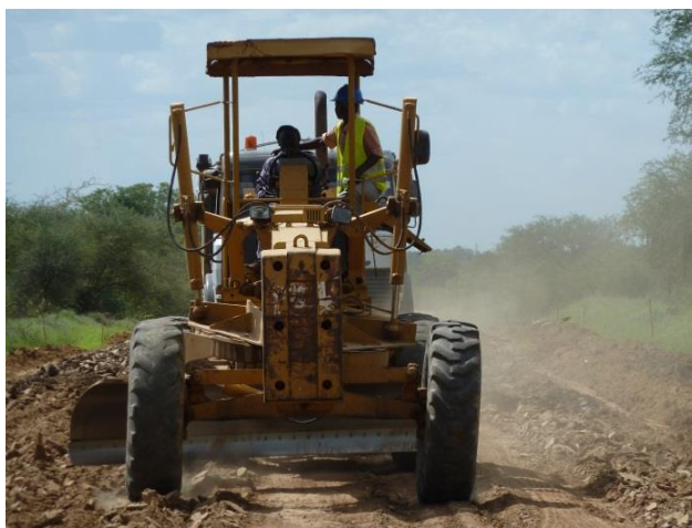
Figure 5.1 – Motor grader used for maintenance of unpaved rural roads, (Image: Intech Associates)
