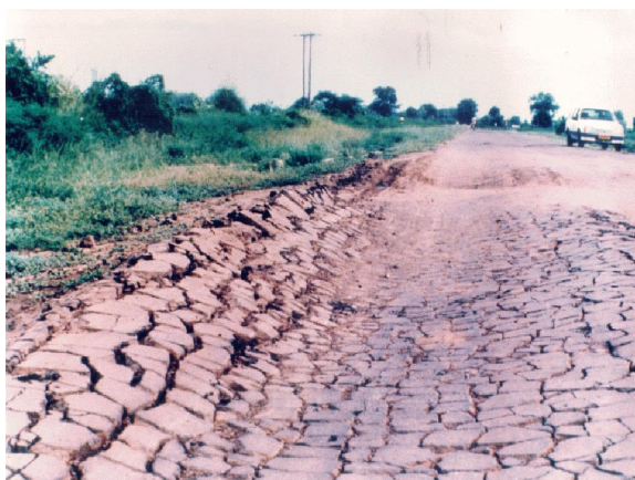
Overloading – causes accelerated pavement deterioration
