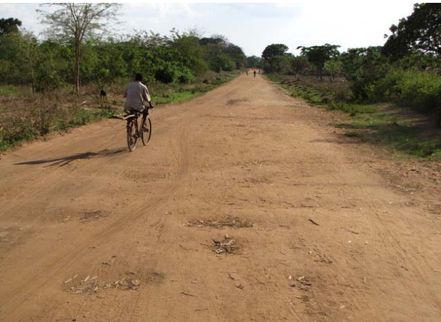
Section of badly rutted and pot holed, gravel section of road in low-lying, poorly drained area
