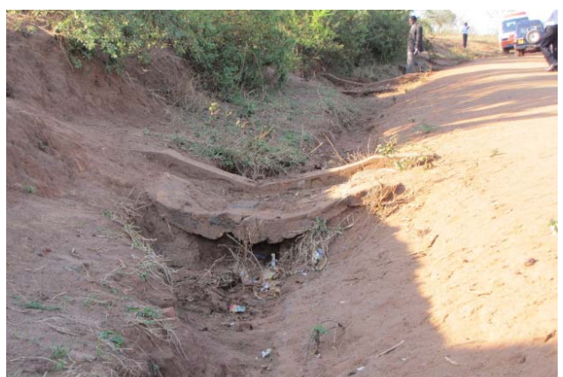
Section of road on relatively steep gradient showing severe erosion of drain downstream of scour check
