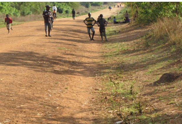
Well formed and drained, gravelled section of road exhibiting significant gravel loss after one year
