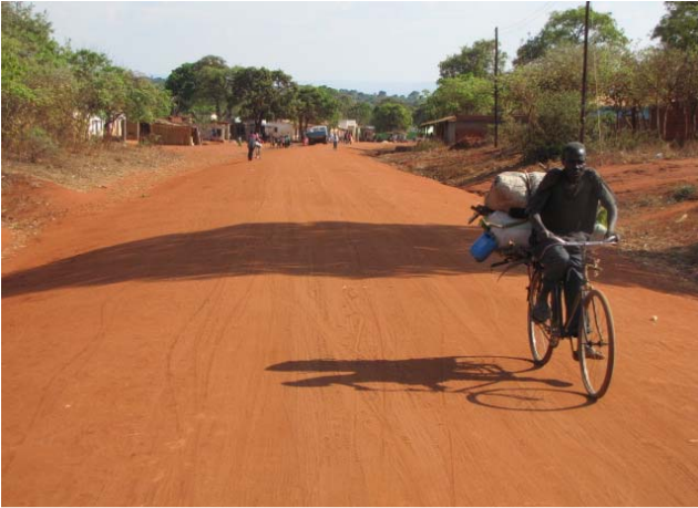
Section of well-formed and drained sandy clay running surface (no gravel wearing course) in good condition near Malingunde
