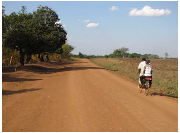
Section of recently graveled section of road in very good condition in reasonably well drained area
