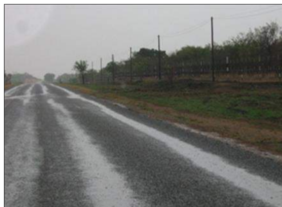
Figure B.4-1: Water ponding in wheel track
