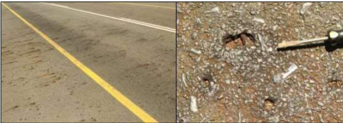
Figure B.2-8: Aggregate loss due to disintegration
