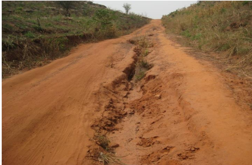
Erosion Caused Gullies On Teiwanya-Sekasua Road Section
