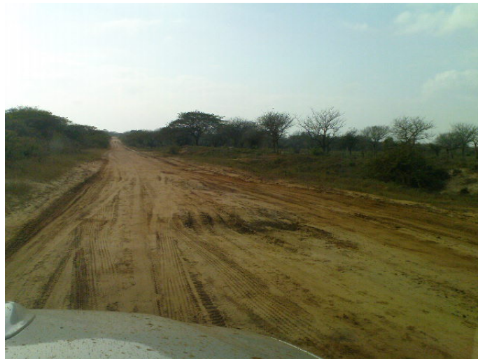
Route No. N221 Boane - Bela Vista - Maputo Province Condition: Poor
