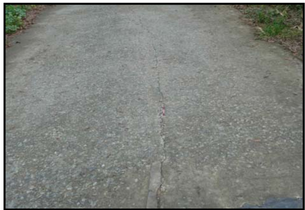
Figure 3.9 TG2-. Single crack running along centre-line of slabs . .
