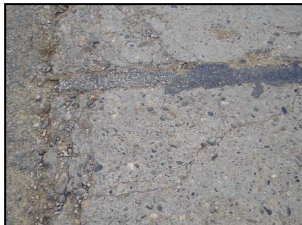
Figure 3.7 TQ(1)-2. Indication of disintegrating poor quality concrete with rounded aggregate. .
