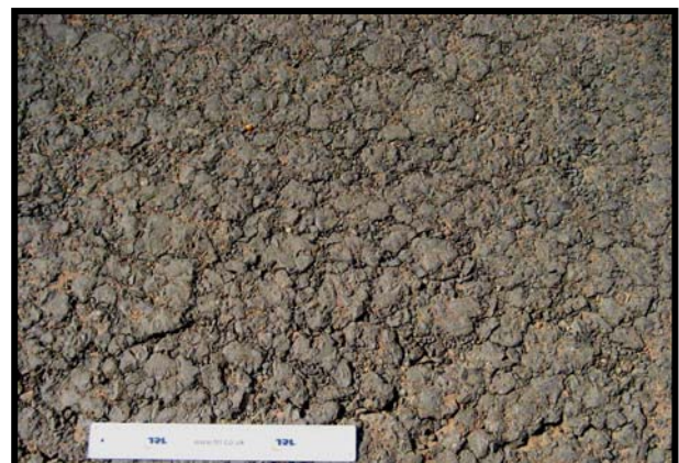
Figure 4.2 .Cracking in PenMac in Ea Soup road DL(3)-2
