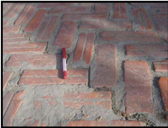
Figure 5.5 Cracks in mortared joints with intact clay bricks (D10)
