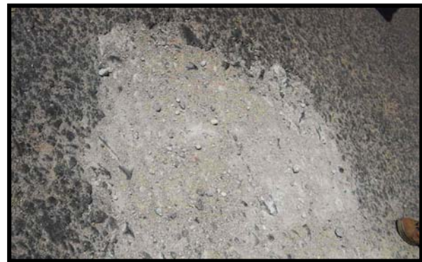
Figure 4.1 .Pothole in PenMac in Ea Soup road DL(3)-2
