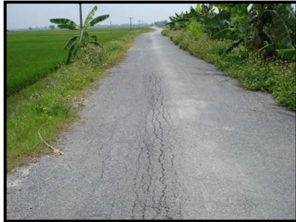
Figure 4.8 .HY(2)-4. Longitudinal cracking associated with probable sub-grade movement
