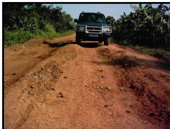
Figure 4.6 .DL(2)-2. Pavement failure caused by excessive traffic overloading
