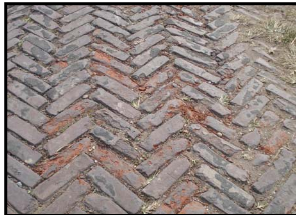
Figure 5.10 Sand joint clay brick pavement HY(2)-2 exhibiting significant seal loss and brick deterioration after 2 years of service
