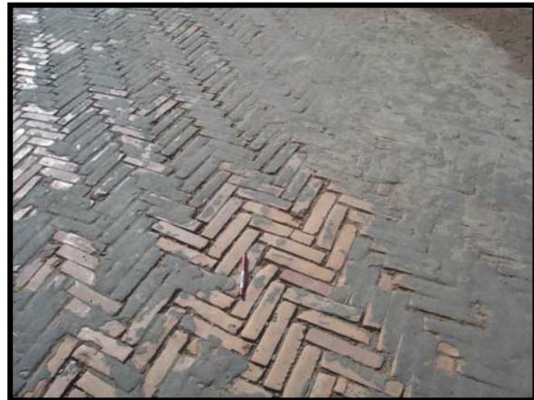
Figure 5.9 Sand joint clay brick pavement (D11) exhibiting significant seal loss after more than 3 years of service
