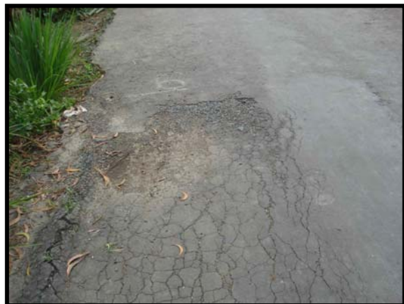
Figure 4.10 .TG05. Potholing probably related to localised strength deterioration in stabilised base
