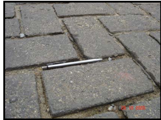
Figure 5.6 Eroded sand joints with intact concrete bricks (H07)
