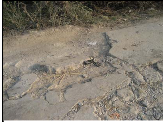
Figure 3.4 Typical final deterioration of concrete slab (non RRST road)
