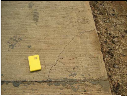
Figure 3.3 Single crack in RRST slab
