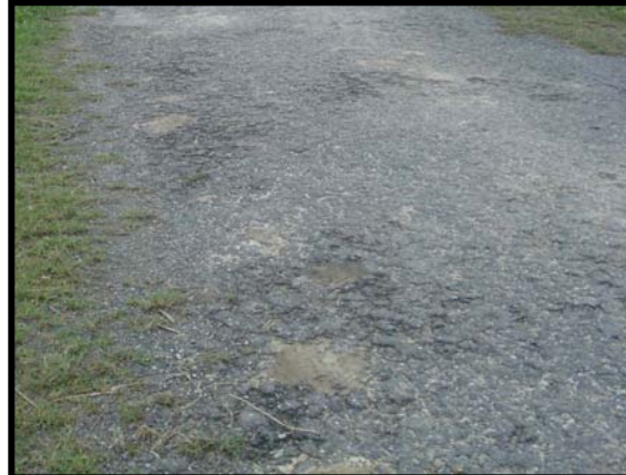
Figure 4.5 .DaN05. Rapid deterioration of surface seal following a number of tropical storms and associated flooding
