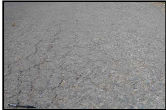
Figure 4.11 .TQ(2)-1. Cracking probably related to recorded weakness in sub-base and sub-grade.
