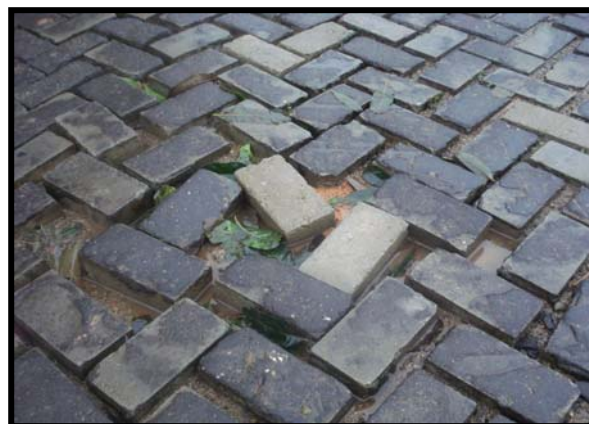
Figure 5.11 Sand joint concrete brick pavement (H07) exhibiting total seal and joint deterioration with consequent loss of pavement integrity. January 2009, following rainy season with intense tropical storms
