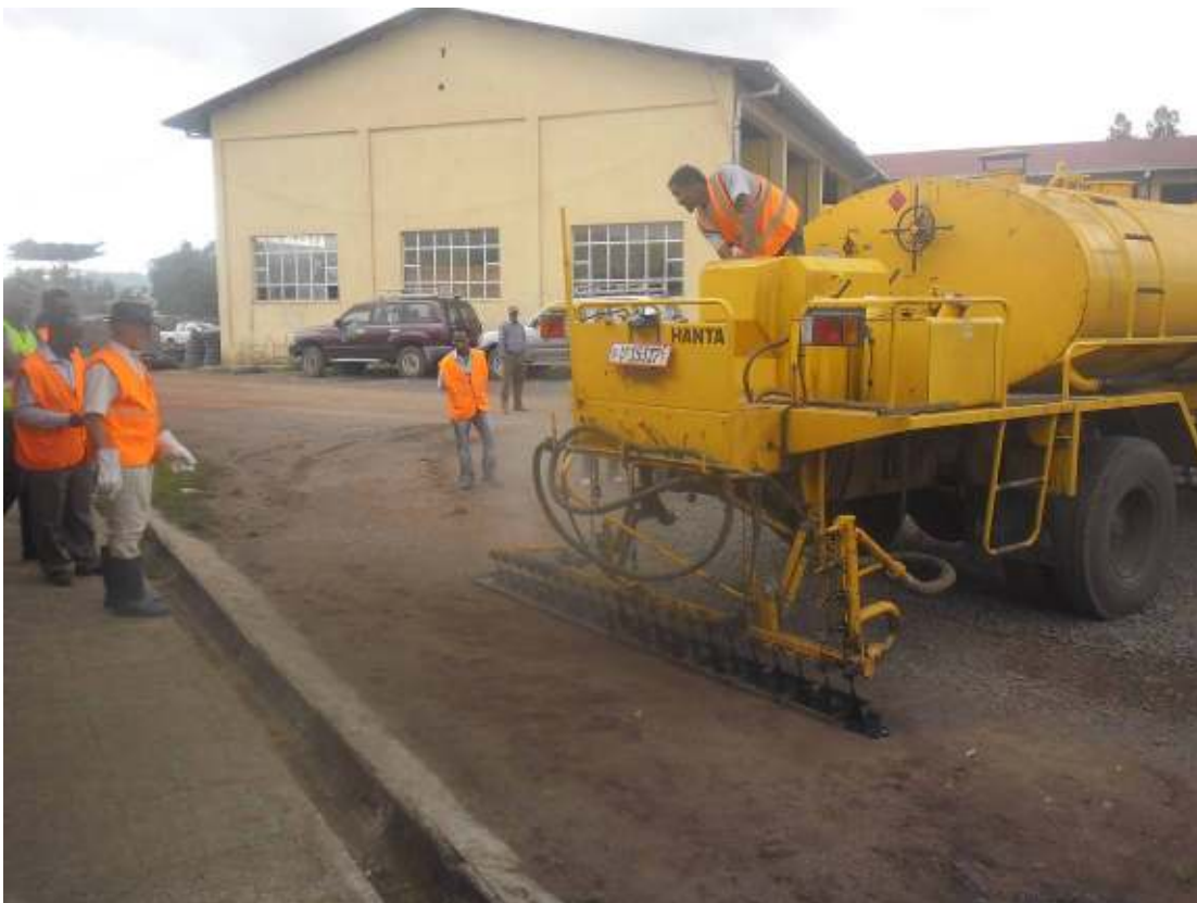
Figure 3-3 Transverse Spray Test
