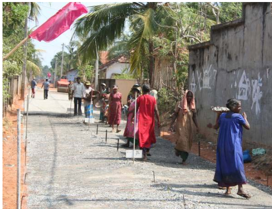
Photo 3: Placing base course using strings, pegs & line levels for layer thickness & camber control
