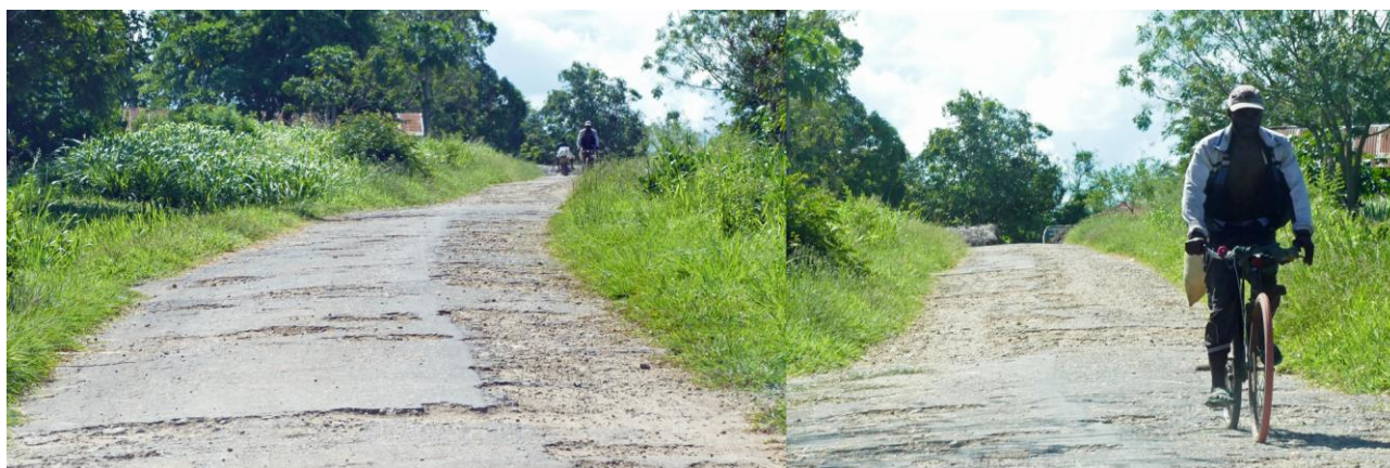
Figure 11 Bituminous slurry seal section on the Bagamoyo road in Tanzania showing deterioration
