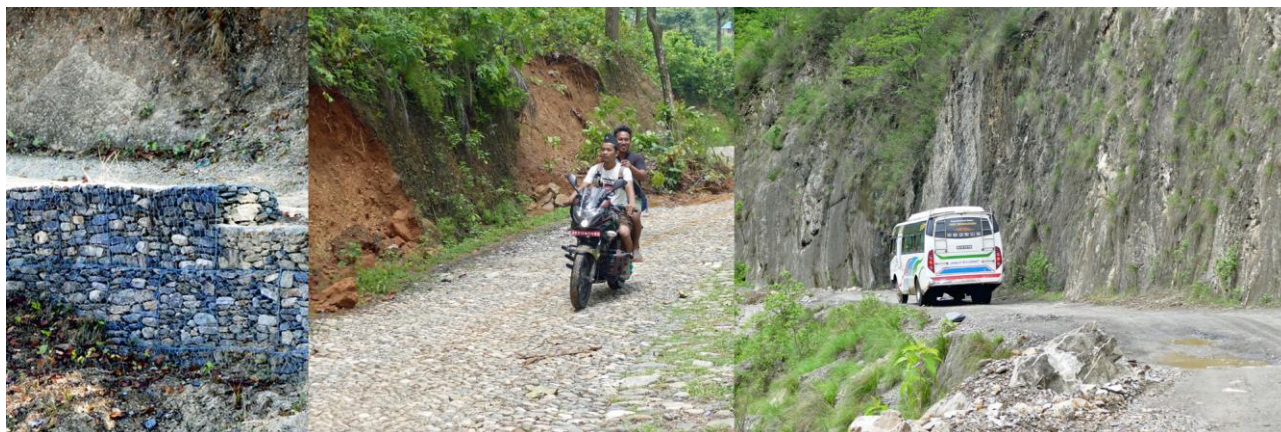
Figure 3 Sections of the two Nepal roads, showing gabion supporting structures, cobblestones and an earth section
