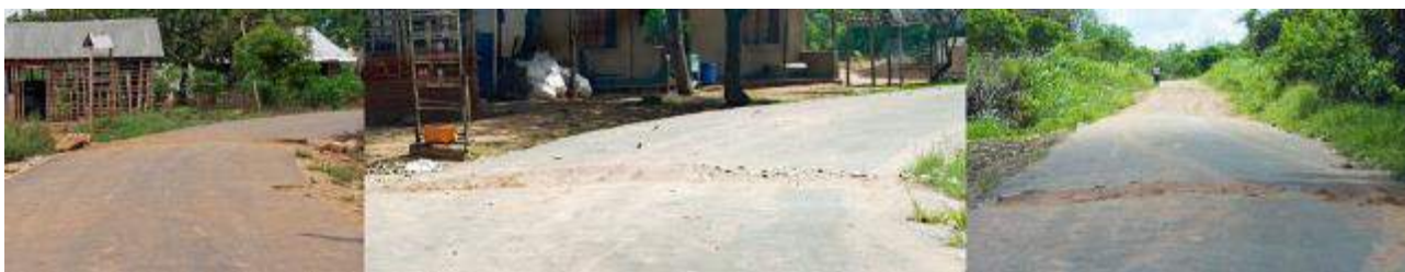
Figure 110 Village attempts at traffic calming on a double sand section in 2015 (left) and in 2019
