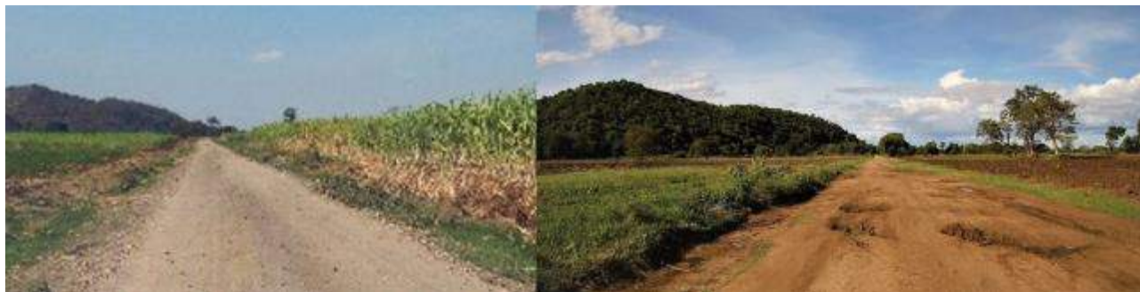
Figure 37 Low-lying section in 2015 at the time of IRAT investments (left) and potholed in 2019 (right)
