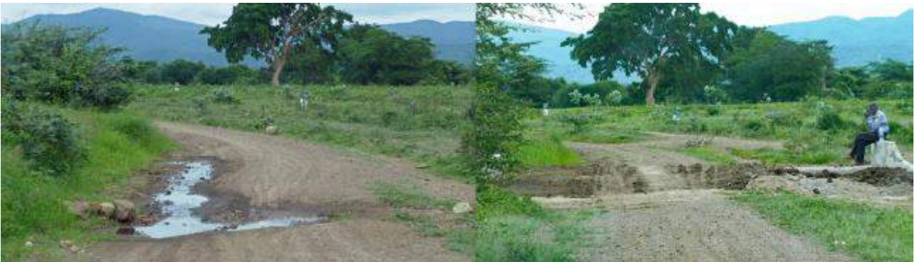
Figure 16 Road within Kaway showing a failed culvert (June 2019, left) and the new culvert (Nov 2019)
