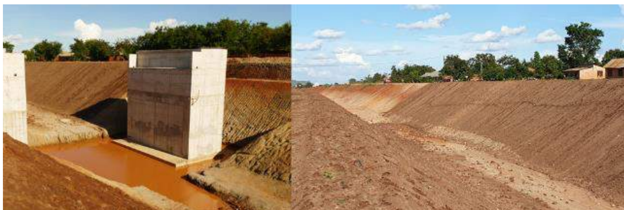
Figure 86 Construction of the new railway causing severance of the first section of the survey road
