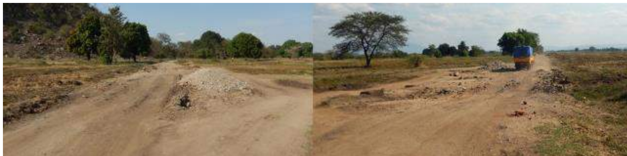
Figure 32 Site of a critical low-lying bottleneck section and failed culvert in 2015 before IRAT investments
