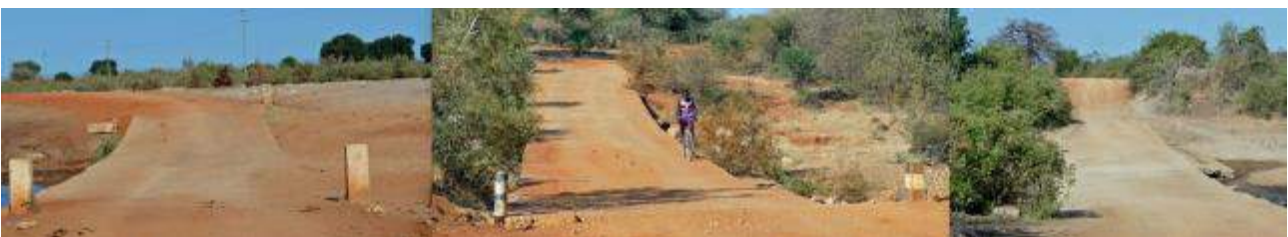
Figure 59 Chigongwe-Chipanga road showing some of the drifts
