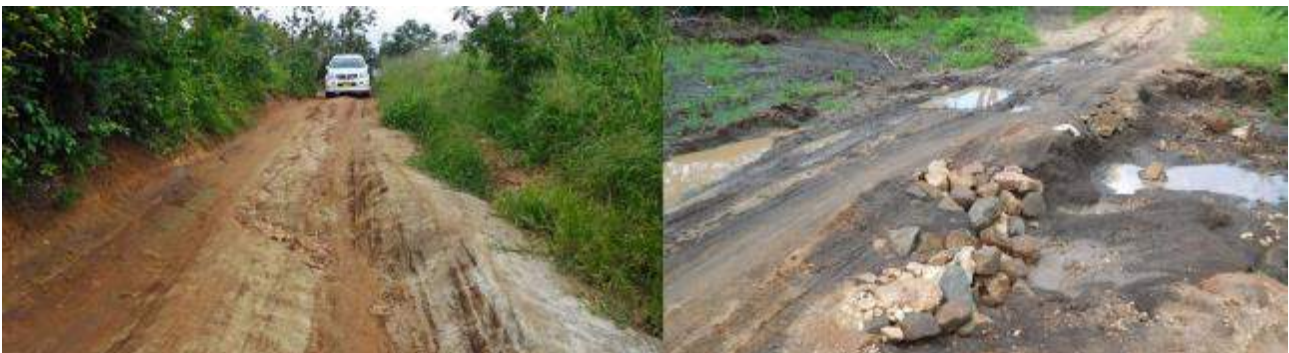
Figure 85 Condition of parts of the road in 2016 showing need for further bottleneck interventions
