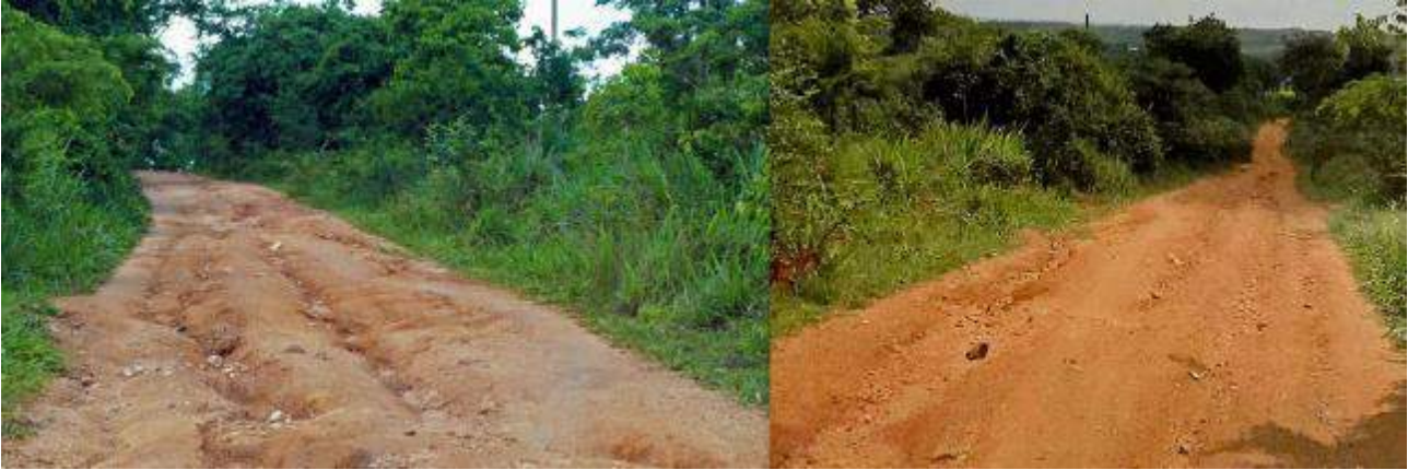
Figure 90 Eroded slopes on the Mikese-Ngeregere road in 2019
