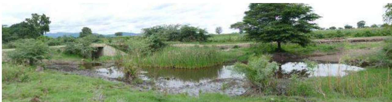
Figure 23 Culvert around 4.7 km showing eroded embankment caused by high water levels after heavy rains
