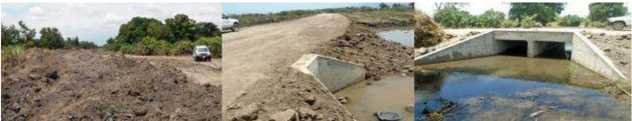
Figure 12 Chekimaji to Kawaya road during construction showing raised embankment and two box culverts
