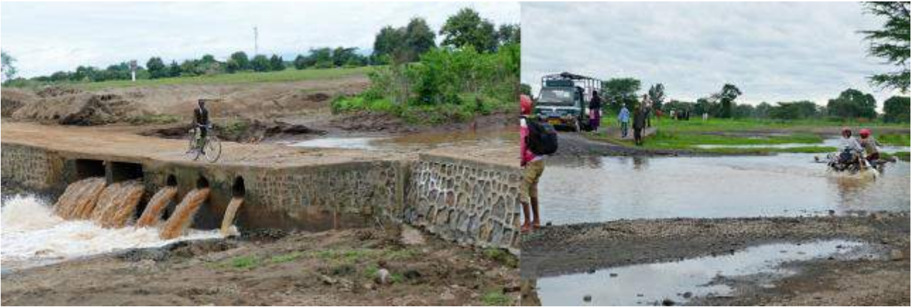
Figure 26 Road from Boma Ng'ombe to Rundugai, showing a drift and a problem water crossing
