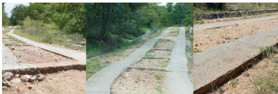
Figure 120 Parallel concrete strips on Morogoro road showing dangerous proud vertical edges
