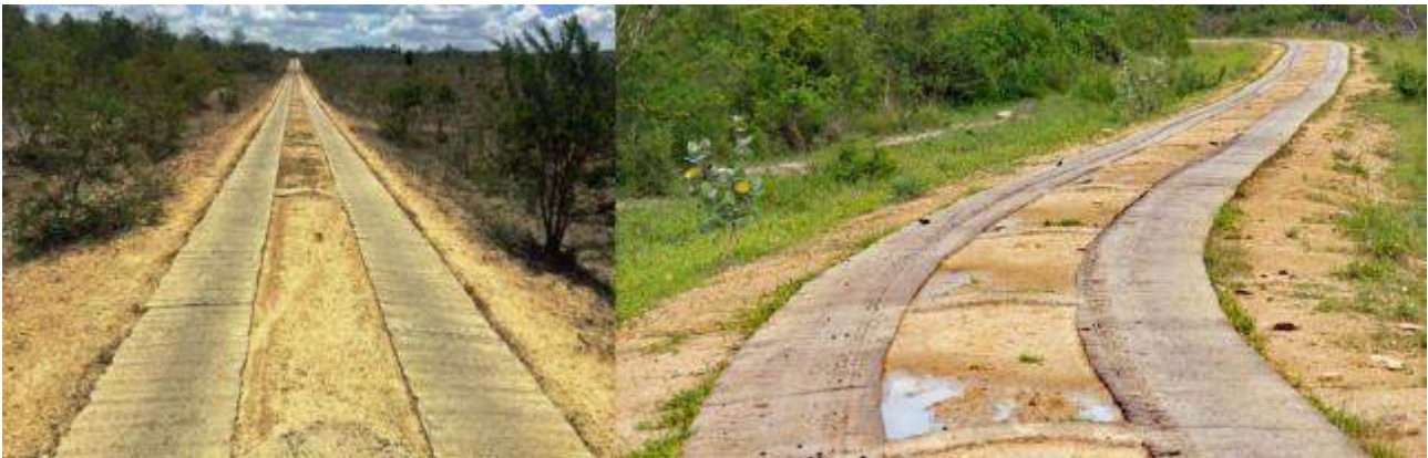
Figure 105 Parallel concrete strip sections in 2011 (left) and in 2015 (right)
