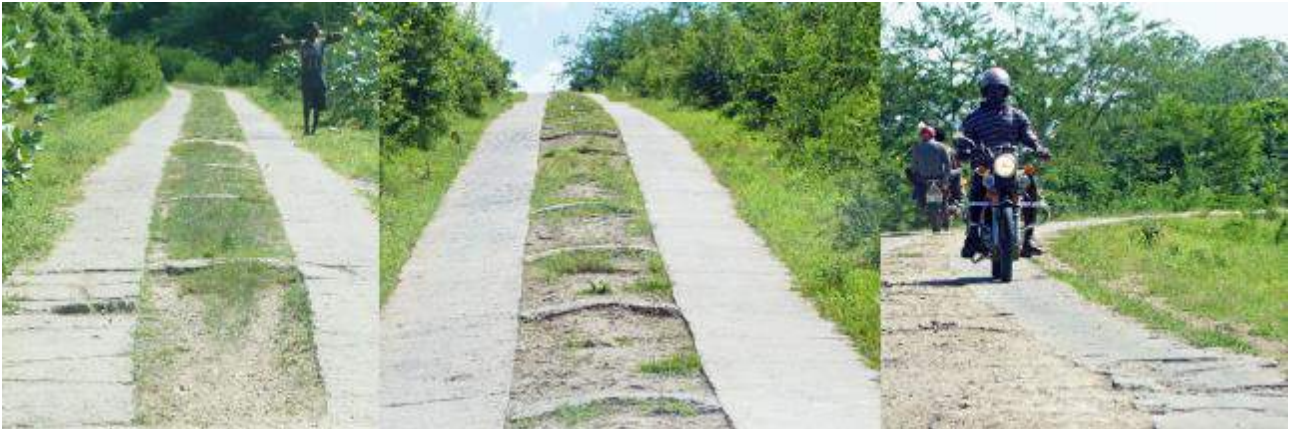
Figure 106 Parallel concrete strips in 2019, showing proud connectors and some sharp edges due to strip damage
