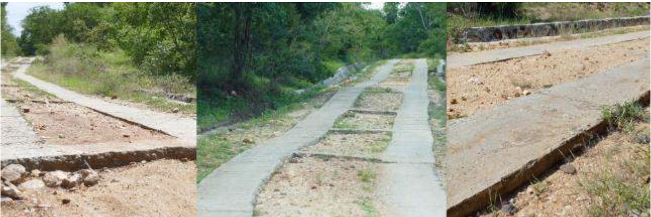
Figure 91 Parallel concrete strips showing proud concrete that is a safety problem for motorcycles
