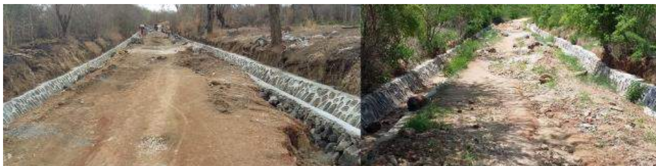
Figure 82 Side drains being constructed during IRAT rehabilitation in 2014 (left) and their state later in 2014 (right)
