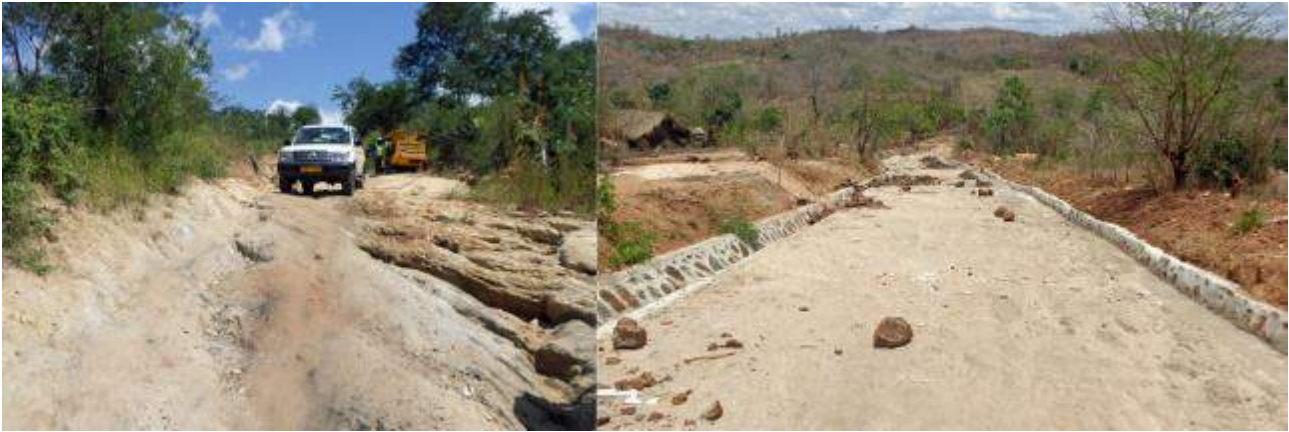
Figure 83 Eroded slope before IRAT rehabilitation in 2015 (left) and subsequent intervention (right)
