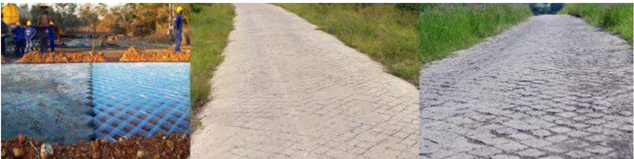
Figure 107 The geocell section in 2011 (left), 2015 (centre) and 2019 (right)
