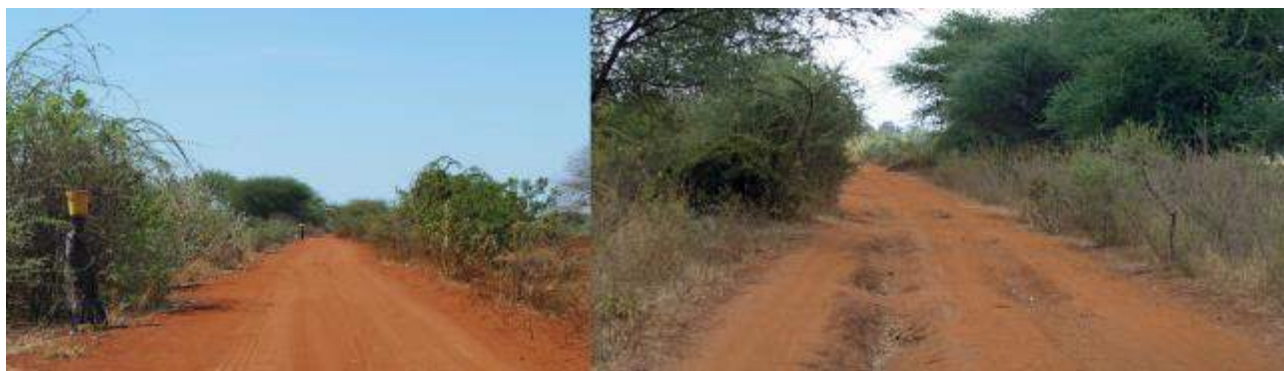
Figure 55 Chigongwe-Chipanga road showing parts that have lost their gravel and shape
