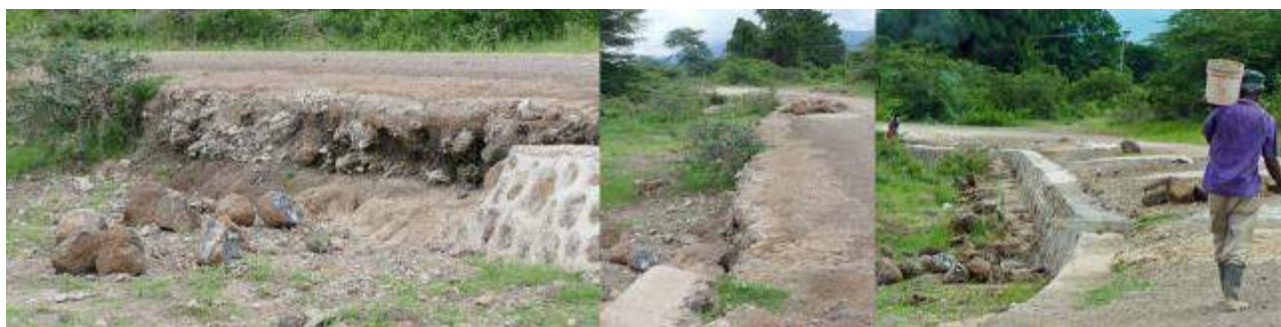
Figure 24 Road embankment near 4.7 km and the final culvert showing water erosion and repair
