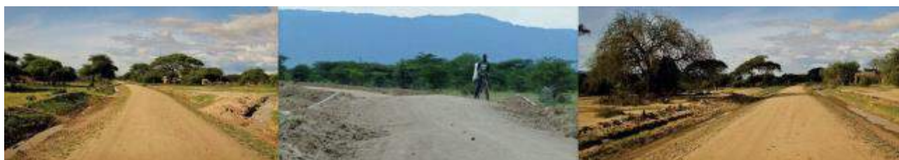
Figure 39 Recently maintained end section showing turnouts, a new culvert and side drains
