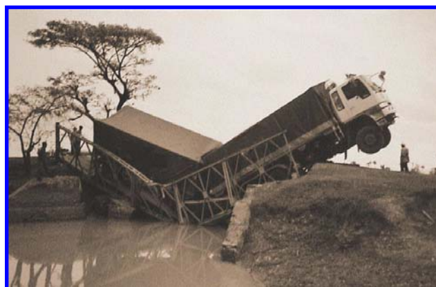
Figure 4 – Overloaded truck damages bridge on a secondary road.
