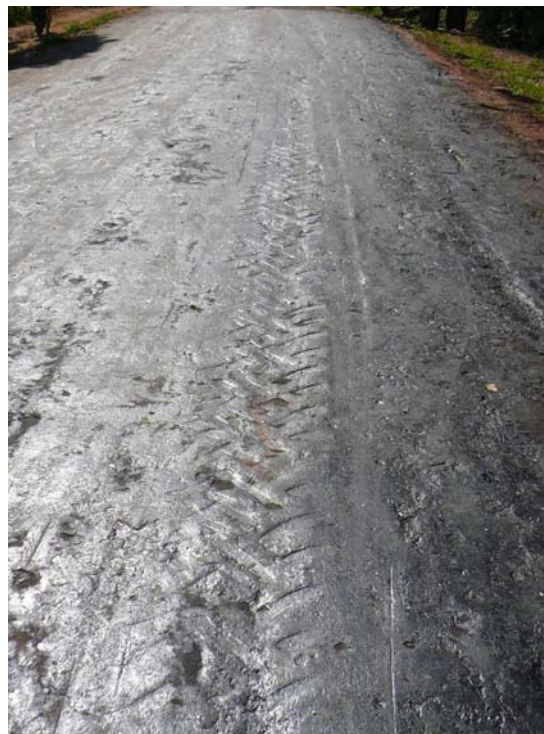
Tractor tyre indentations in the poorly compacted base
