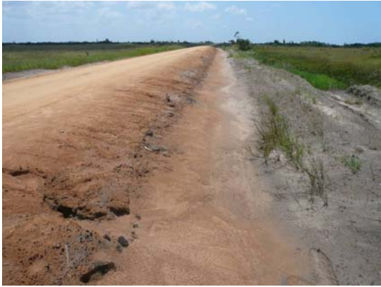
Lateral erosion of the constructed embankment
