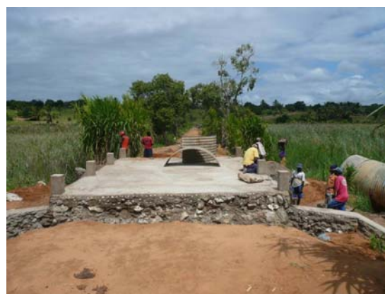
The Rio Cudingene crossing with the bridge in the foreground and the replaced culvert pipes to the right
