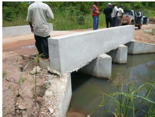
Low wing walls which lead to the erosion of surfacing materials
