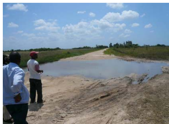
Site of ponding water on the coastal flood
