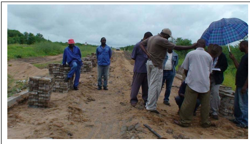
Block paving failures on Macaritane Chicualacuala Road
