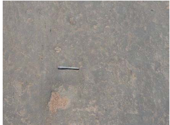
Section 7: Potholes, bleeding and surface detail
