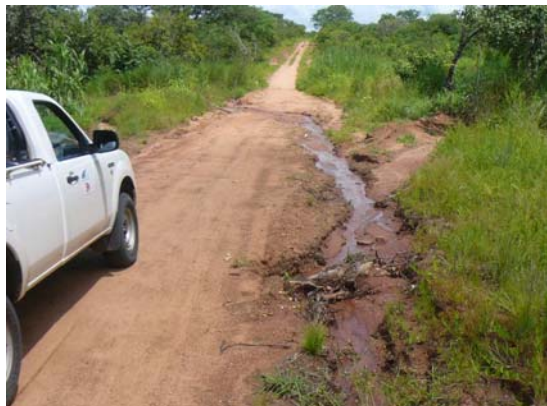
Section of road in need of repair and a new structure
