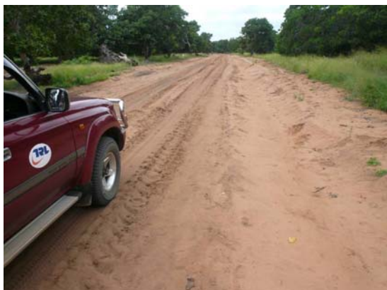
Completed formation which is rapidly collapsing
