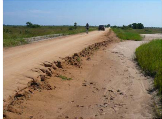
Side drain erosion of the constructed embankment
