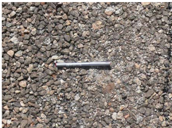
Crushing of Cape seal chippings
