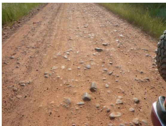
Rough surface of the original road
