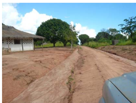
Section of formation degrading without the protection of a gravel surface
