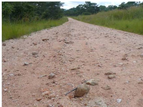
Rough road surface
