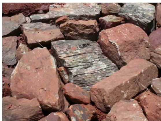
Stone placement – uncompacted soil and loose packing
