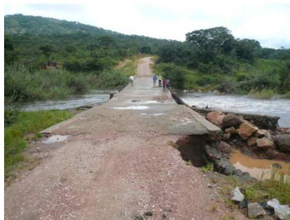
Downstream erosion of improved Rio Nhimbe structure
