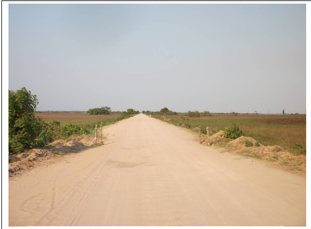
Figure 4-3 Culverts needing extension
