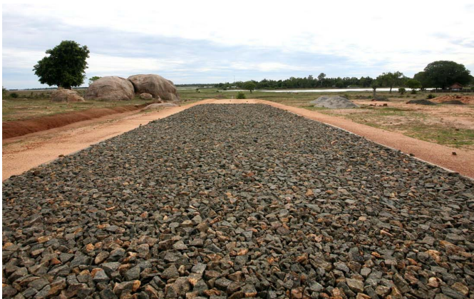
New road constructed in Sri Lanka with SEACAP support linking communities to social and economic opportunities
