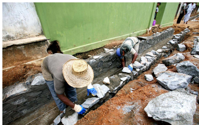
Local workers building gutters for the Community Access Program in the town of Ampara, Sri Lanka
