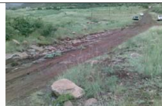
Typical rural road infrastructure used by rural public transport operators observed in Makhuduthamaga area
