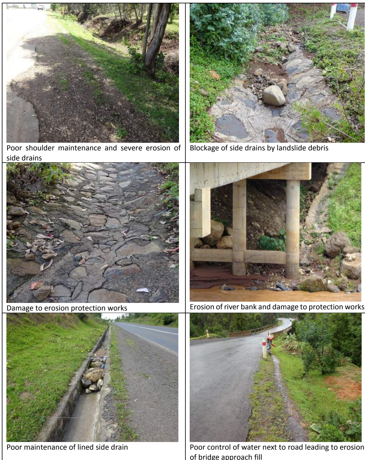
Figure 2 Some defects observed on the Butajira to Gubre road
