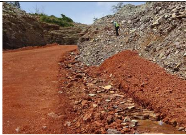
Slope instability problems due to overblasting
