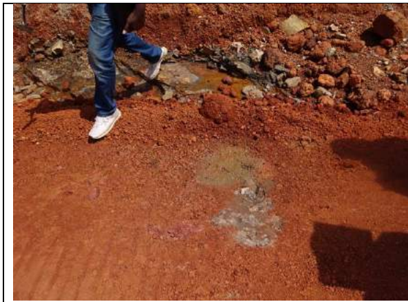
Seepage of water through gravel road from below – rocky subgrade in cutting
