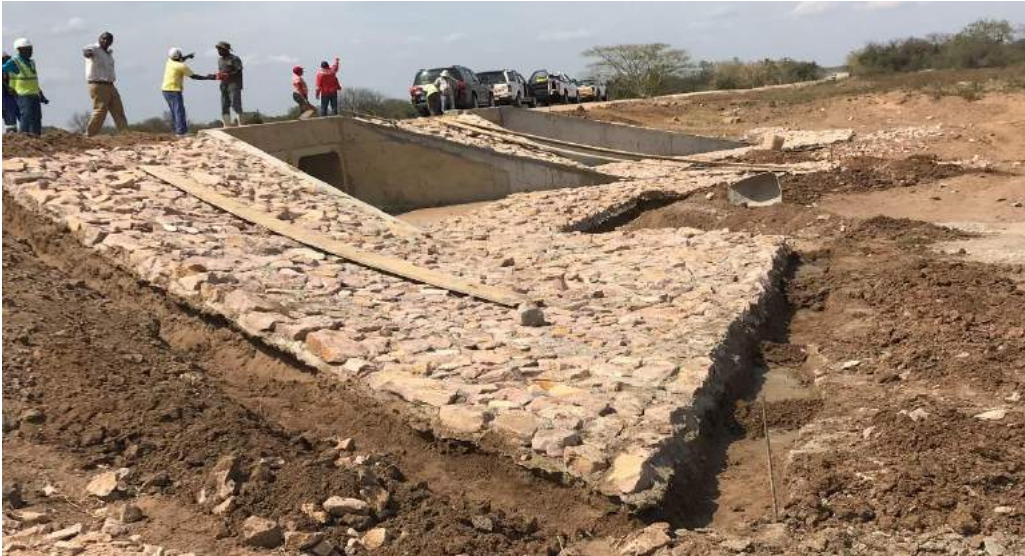
Figure 1.20b Erosion protection construction (stone pitching and beam) for existing culverts at km 43)
