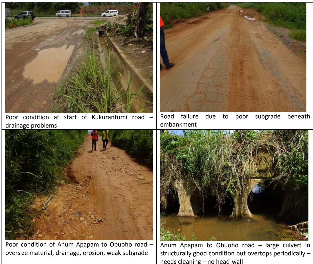
Figure 3 Some defects observed on the inspected roads
