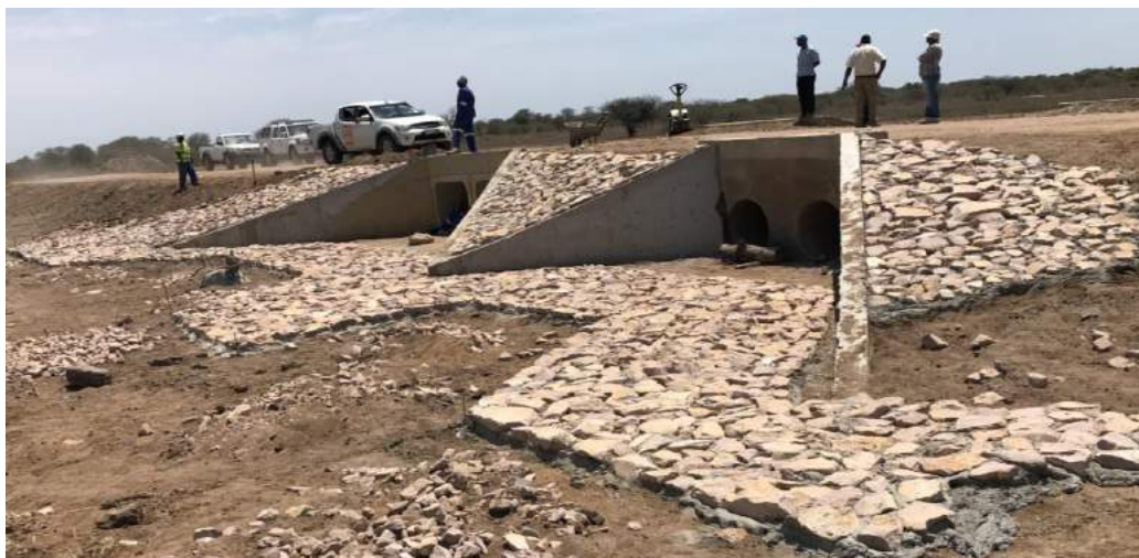
Figure 1.20a Erosion protection construction (stone pitching and beam) for existing culverts at km 43)
