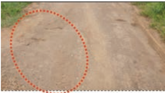
3: Poor: Poor shape and seriously restricts water to run off the road surface into the roadside drains; severe erosion of shoulder
