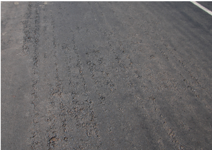
Photograph 2: Poor transverse distribution - high application rate
