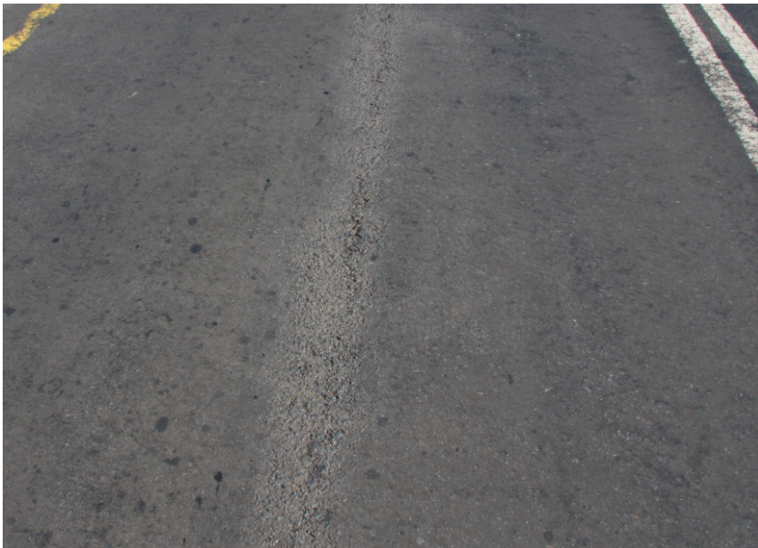
Photograph 8 Poor longitudinal joint (not on centre line)
