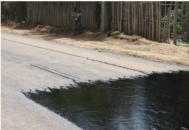
Photograph 11 No transverse joint protection
