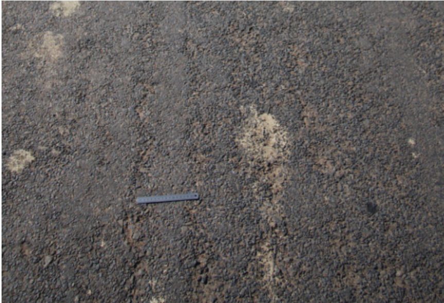
Photograph 1: Poor transverse distribution – low application rate
