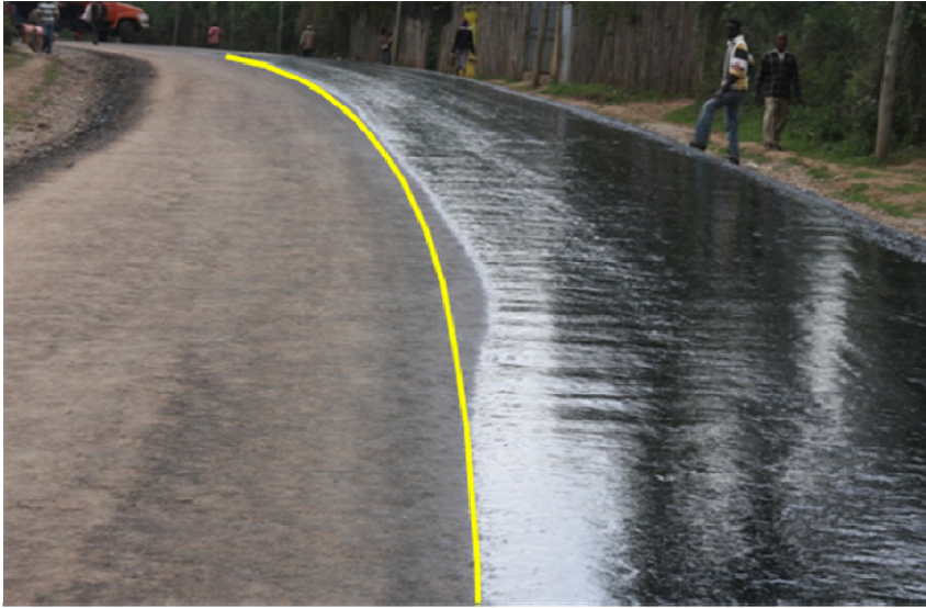
Photograph 7 Impact of no stringline placement
